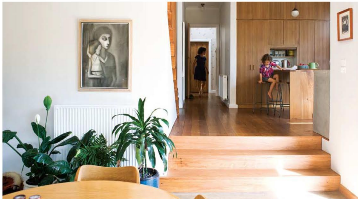
Original flooring was removed for recycling and replaced with recycled Blackbutt, insulated underneath to prevent drafts.
